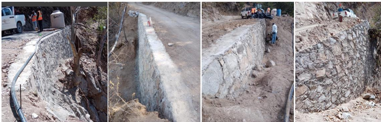
Figure 4-3: Access Road Stability Retaining Walls Built by Community Members with Oroco Financial Support
