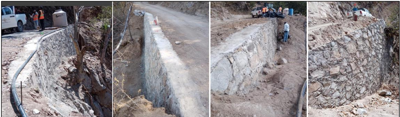
Figure 4-3: Access Road Stability Retaining Walls Built by Community Members with Oroco Financial Support
